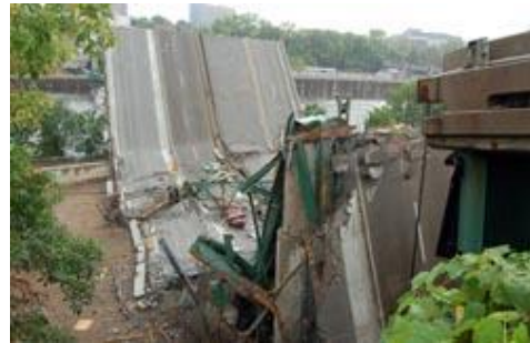
Before its collapse last year, the Interstate 35W bridge in Minneapolis was part of the one quarter of the nation's bridges that are considered either 'functionally obsolete' or 'structurally deficient'.
