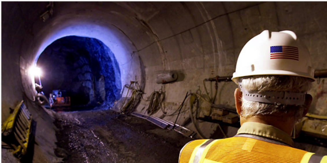
A worker near the end of a tunnel under 63rd Street in Manhattan that will, at long last, connect the Long Island Rail Road to Grand Central Terminal.
